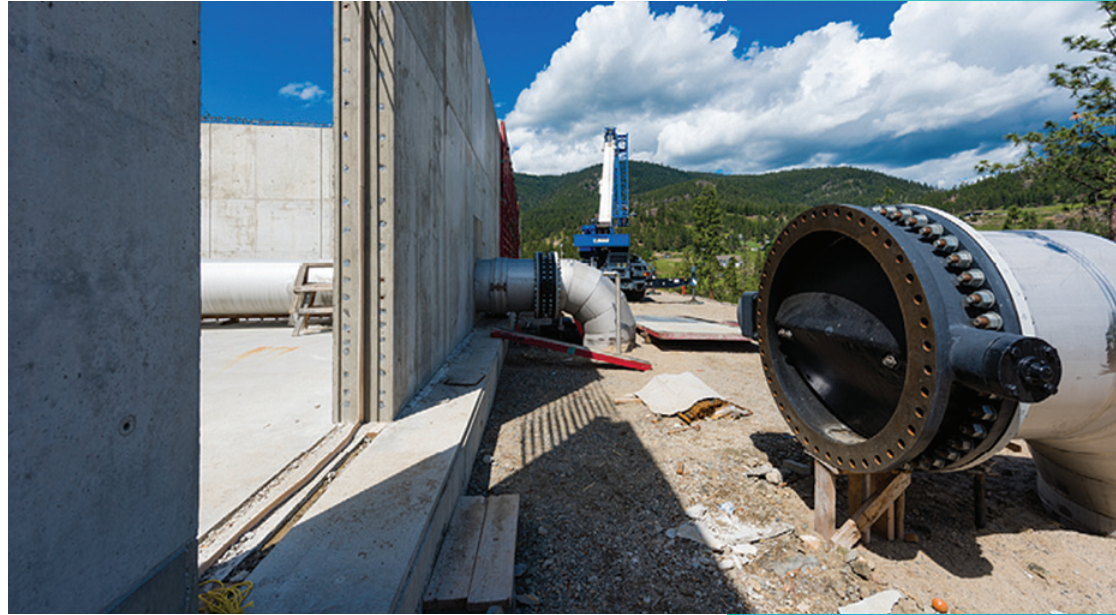
Pipe connection to the Rose Valley treated water reservoir. Credit: City of West Kelowna
